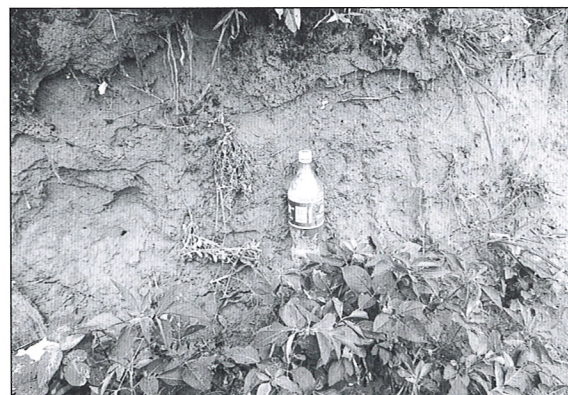
Figure 3a. Erosion caused by high flow velocity at the outside of the meander bend
